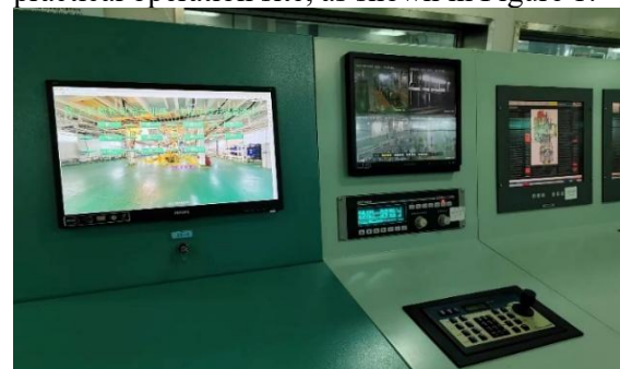
Figure 1. Online Simulation Operating System Installed on the Control Console
